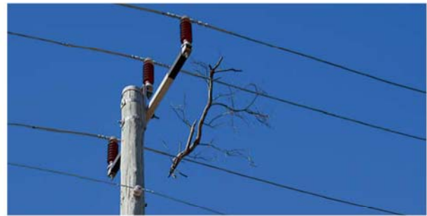
Fallen branches often cause temporary faults on powerlines
